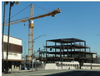
COULD THIS OFFICE PROJECT AT ROBERTSON REMAIN HALF COMPLETED?— 8767 Wilshire Boulevard lost its construction loan in September 2009, according to the project's attorney. If it does not secure financing the project will be left mid-construction.
